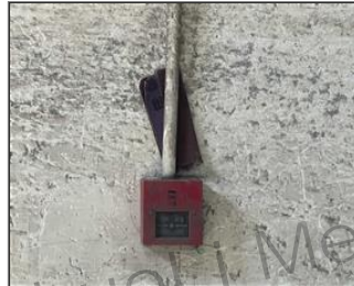
Photo of fire safety equipment fire alarm.JPG
