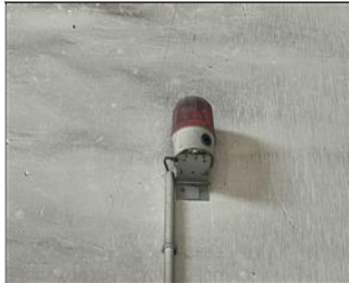
Photo of fire safety equipment fire alarm light.JPG
