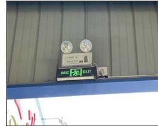
Photo of fire safety equipment exit and emergency light.JPG
