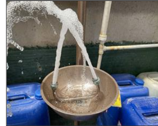
Photo of chemical storage room (if applicable) eye washer.JPG
