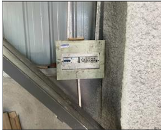
Photo of non-conformity NC-no cover.JPG
