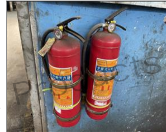
Photo of fire safety equipment fire extinguisher.JPG
