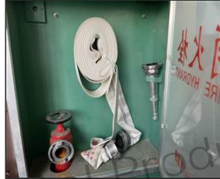
Photo of fire safety equipment hydrant.JPG
